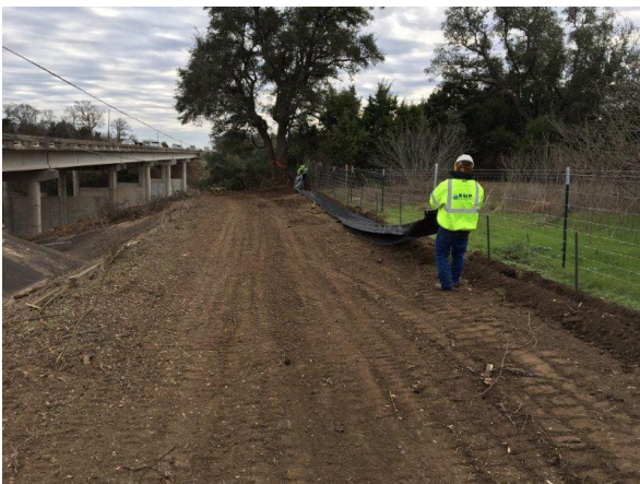
5. BMP Specialists Installing Silt Fence North of Onion Creek East West of FM 1626
