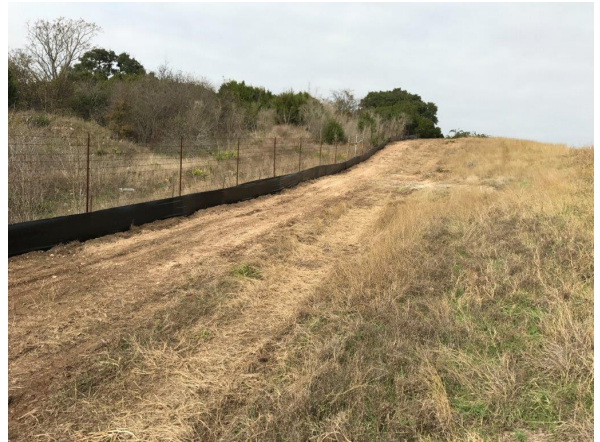
2. Silt fence installation on west side of FM1626 south of Onion Creek
