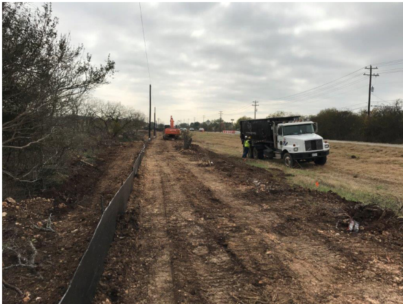
3. Brush removal from east side of project from RM 967 to Oyster Creek
