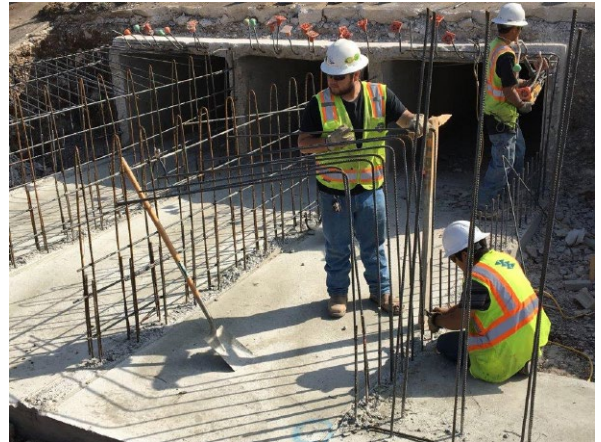
2. Sterling Installing Rebar for Wall of Existing Box Culv N of Oyster Creek
