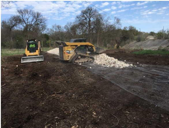
3. BMP Specialist Installing Rock Filter Dam on S Bank of Mustang Creek
