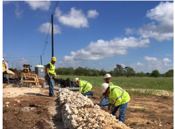
2. BMP Installing Rock Filter Dam at Box Culv N of Oyster Crk
