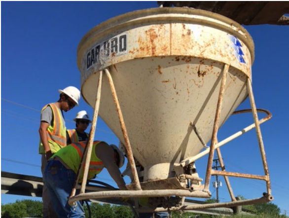
1. Sterling Pouring Concrete for Proposed Box Culv N of Oyster Creek Dr
