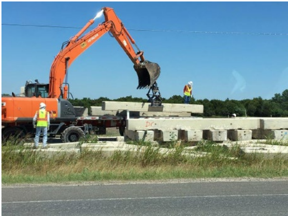
3. Sterling Unloading Lo-Pro Barrier N of FM 2770
